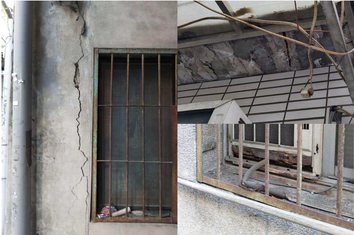
Figure 14 - Highlights from a quick structural survey of a single block. Deep cracks, water damage, exposed rebar, poor wiring. Every building of this era had major maintenance issues clearly visible from the street.
